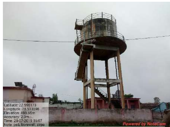
Figure 3-86 : Water Tank, Jhirpa
