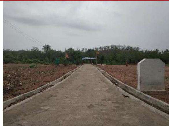
Figure 3-112 : Road with Both side drains, Tawa
