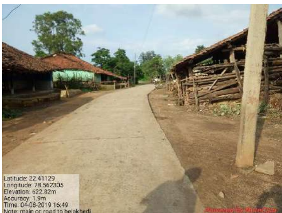
Figure 3-115 : Road without drains to Belakhedi
