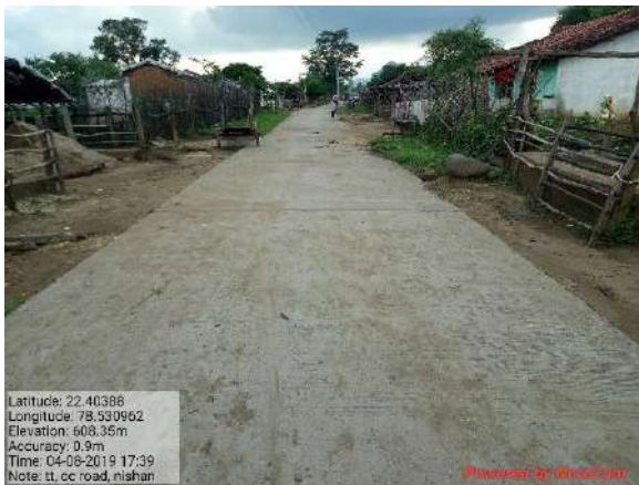
Figure 3-107 : Road without drain, Nishan
